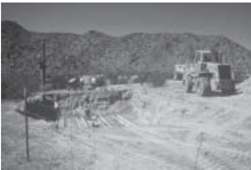
Figure 3—Guzzler under construction in the North Maricopa Mountains Wilderness. Photo courtesy of Bureau of Land Management.
